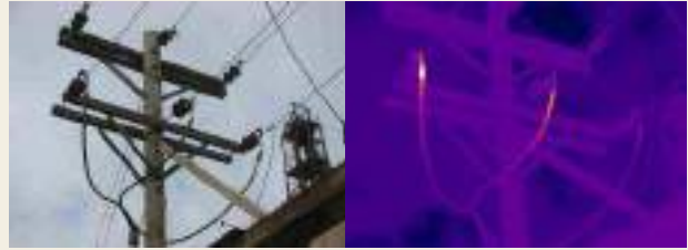
Distribution line faults
